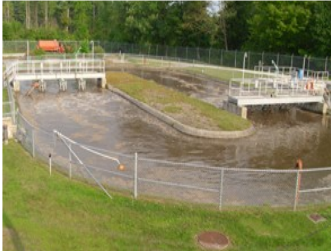
The upgrades net excellent effluent results.
