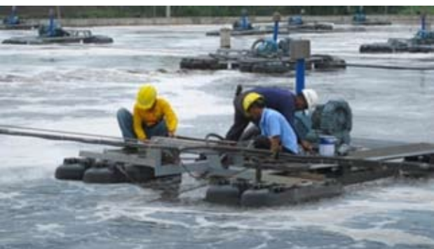
Three men easily perform routine maintenance on the aerator in the field.
