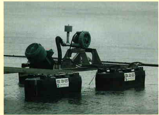
Aerators driven by energy-efficient motors, which are activated by oxygen sensors, help reduce energy use by nearly 60 percent at Astoria's wastewater treatment plant.
