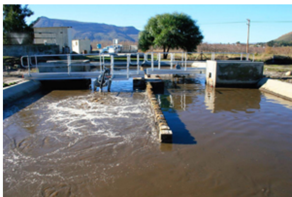
New aerators help meet regulations and save energy
